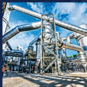
Fabrika sumporne kiseline i topionica bakra, Bor, Srbija Sulfuric Acid Plant and Copper Smelter, Bor, Serbia
